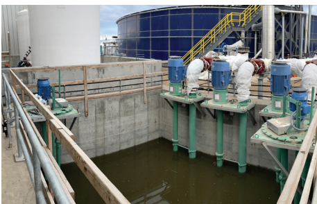
Pumps and Turbo mixers
